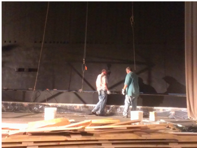
Dave Masserant and George Stampelis on the floor attached the winch cables making sure she was raised and leveled properly while two in the attic worked the winches.
